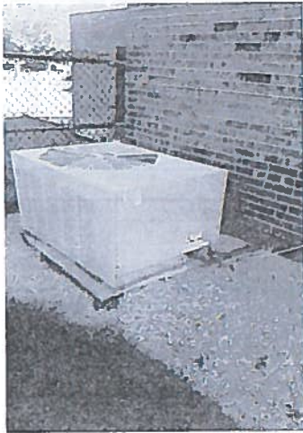
Image 5 – Outdoor Air Cooled Condensing Unit
