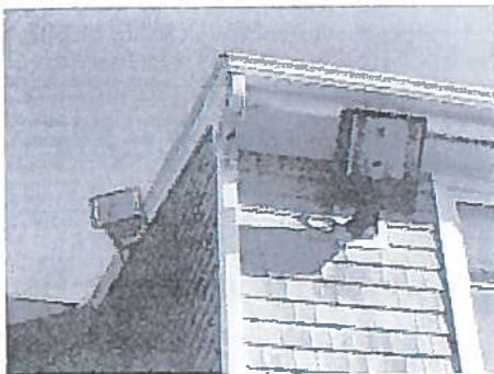
Image 7 – Building Mounted HID Flood Lights
