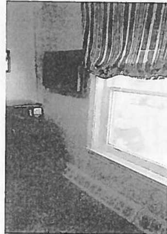
Image 7 – Wall Air Conditioner
