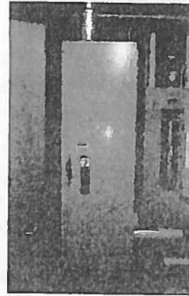
Image 9 – Automatic Transfer Switch
