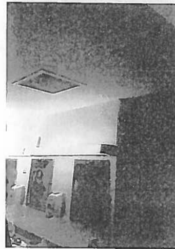
Image 8 – Toilet room Exhaust
