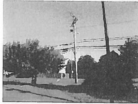
Image 1- Pole Mounted Overhead Service
